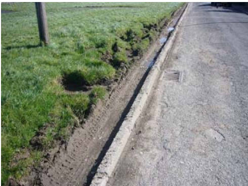
Vehicles are beginning to erode this grass verge.
