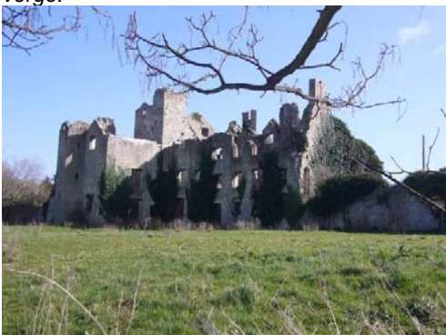
Boverton Place is in need of stabilisation and repair.
