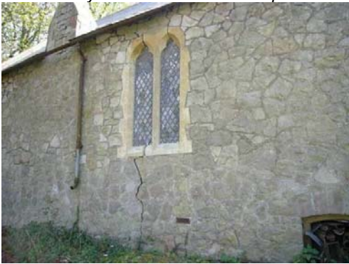
Cracks in the church's masonry are a cause for concern.
