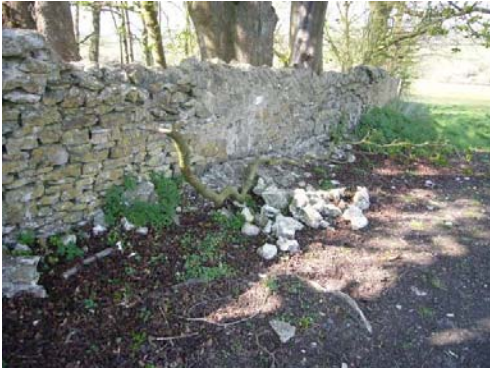
The churchyard wall is in need of repair.
