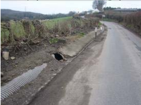
The culverted stream beside the approach from Greenway is in need of repair.
