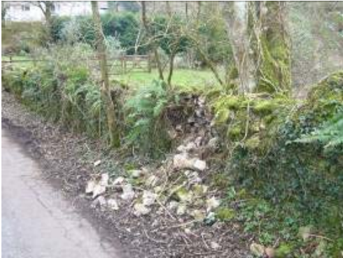
Stone walls have collapsed in places.
