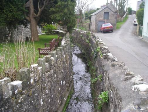
The walls to the Church form part of a culvert to the Ogney Brook.
