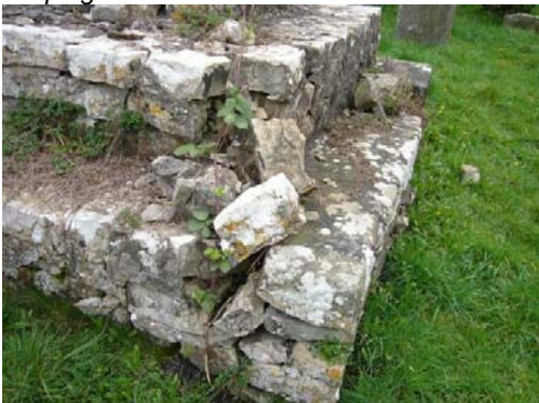
The stone base of the churchyard cross is in need of remedial works.
