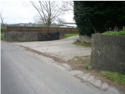
The brick retaining walls beside the entrance to the two modern dwellings are out of keeping with the area.
