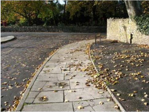
Poor quality pavements in Vennwood Close.
