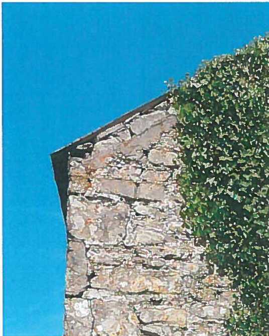
17. The line of the original barge-boards can be seen at the verge of the roof
