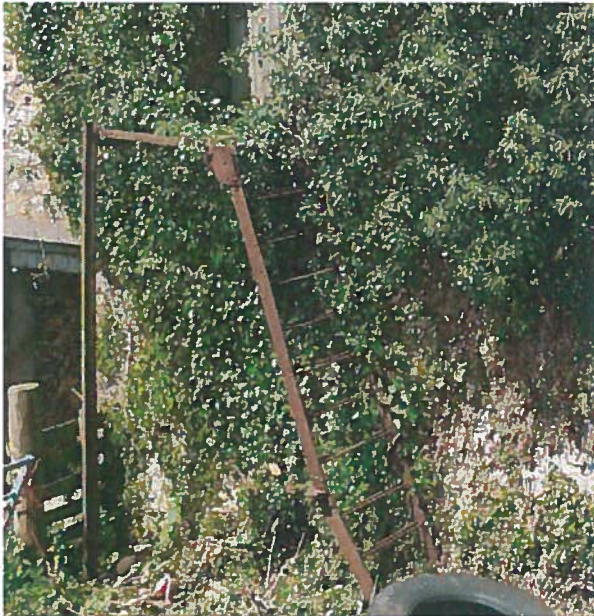
12. The upper door is accessed by a steel staircase, now in rather fragile condition.
