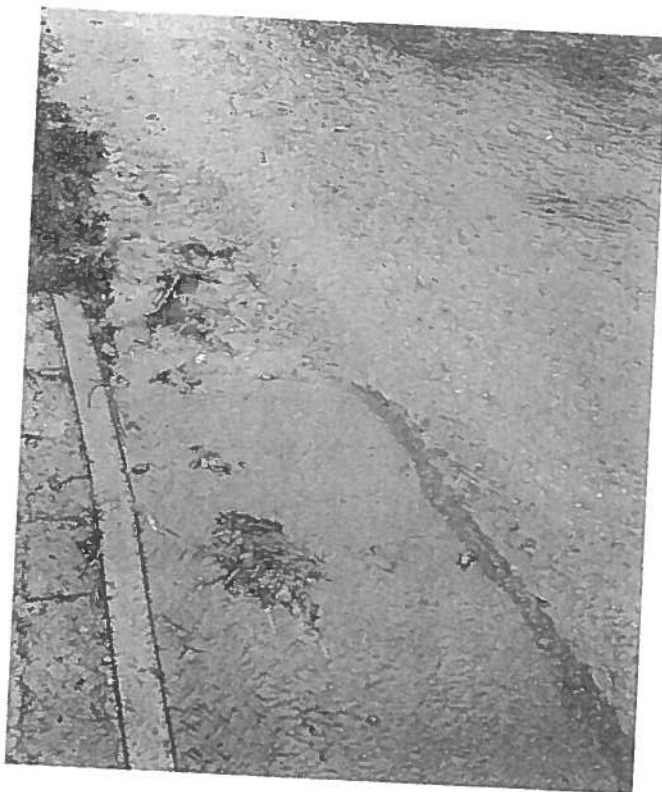
Pic 3 - A close up picture of water running down St Lythan's Road during a medium rain event.
