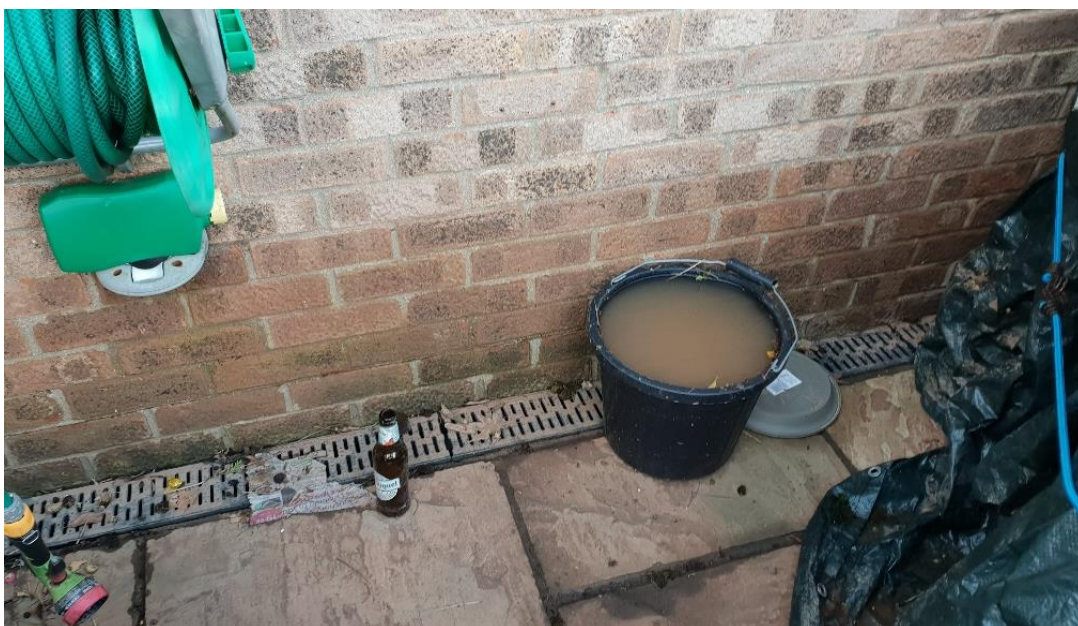
Figure 7-5 Image of external property flood mark within the Swanbridge Grove investigation area (image received from resident completed flood report)
