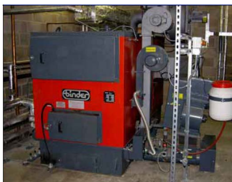
Example 7: Wood Chip Boiler
