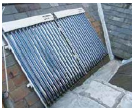
Figure 32: Solar Thermal Collectors Located within Hidden Roof Valley (Source: Cadw)
