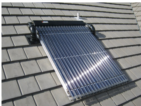
Example 3: Solar Thermal Panels
