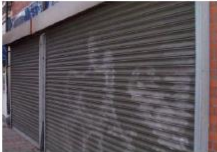
Figure 14: Example of Inappropriate Shutters
