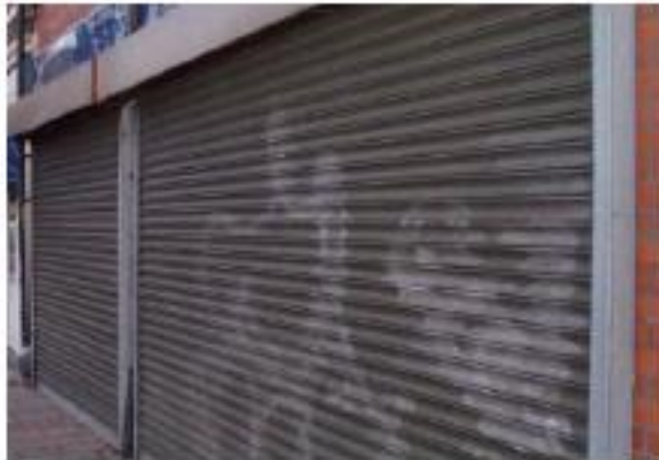
Figure 14: Example of Inappropriate Shutters
